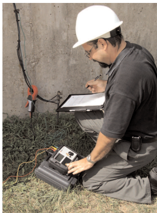
Using ART method with the DET3TC to test commercial ground without disconnecting the system
